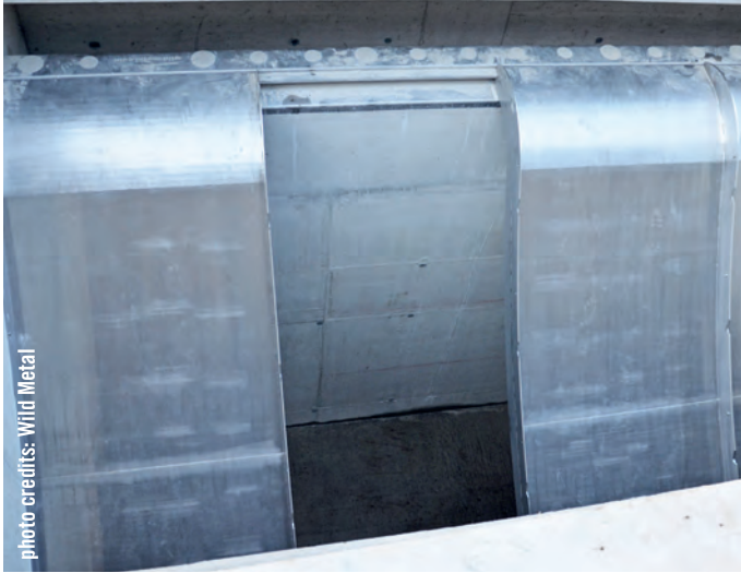
20 modules of the Grizzly Optimus lined up in series produces Europe's biggest Coanda rake with a width of 25 m: at the St. Leonhard power plant in the Pitz Valley. (AT) The absorption capacity totals 4,000 l/s.
