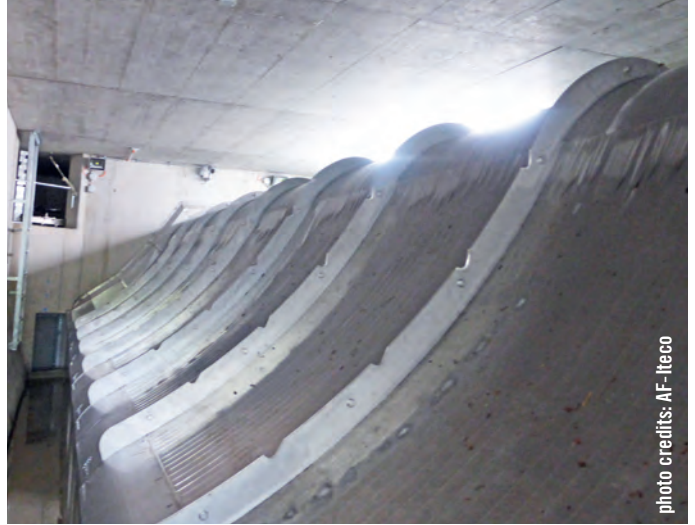
Steineraa PP - Schwyz (CH): The absorption capacity of the Grizzly at Steineraa PP is 1,250 l/s. Thanks to the efficient Coanda system, the people responsible for the project were able to save on the construction of a sand trap.
